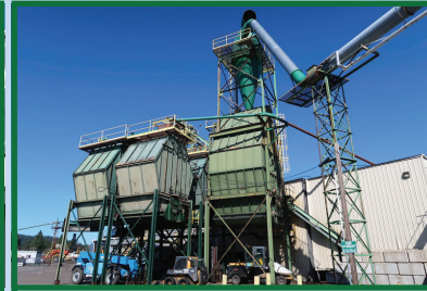
(2) 30-UNIT CHIP BINS
