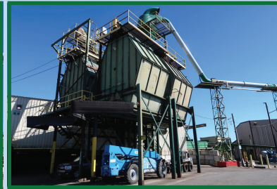
(2) 30-UNIT SAWDUST BINS
