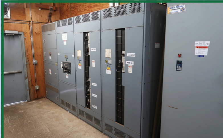
SQUARE D 2,000 AMP 4-SECTION MAIN
