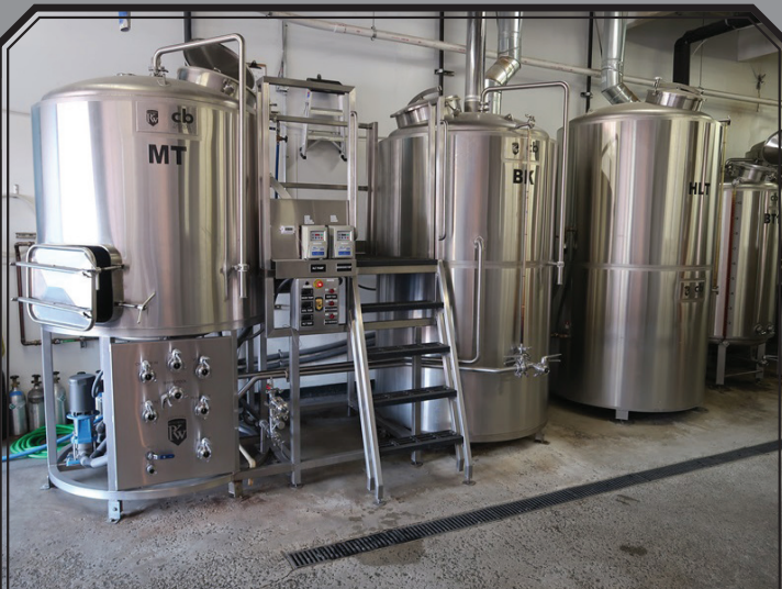
2014 PORTLAND KETTLE WORKS 10 BBL 3-VESSEL BREWHOUSE
